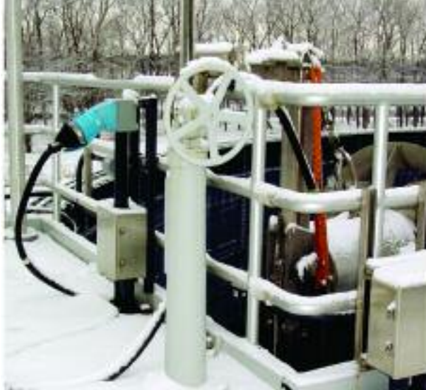
Connection to a Sludge Mixer in a Holding Tank
