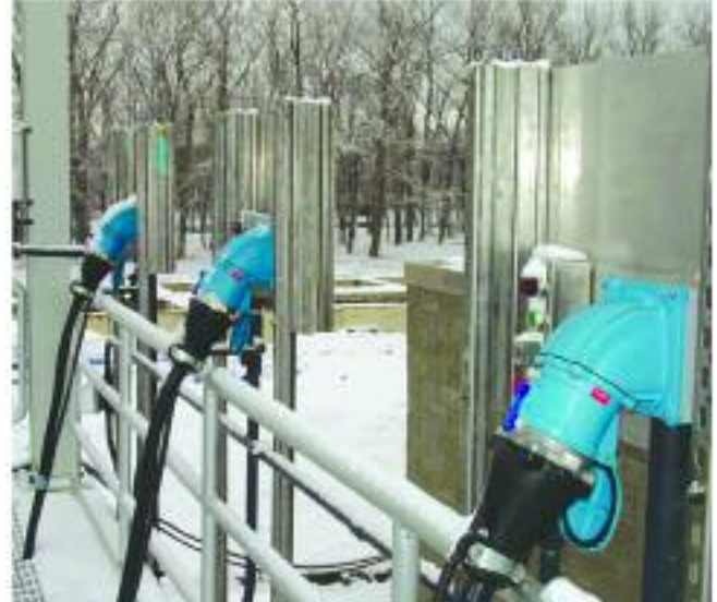
Connections to Submersible Pumps for Effluent Water
