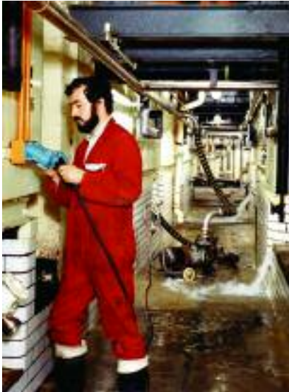
Portable pump connection at a beverage plant
