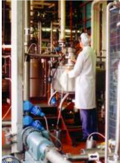
Electrical connections production area - chocolate factory
