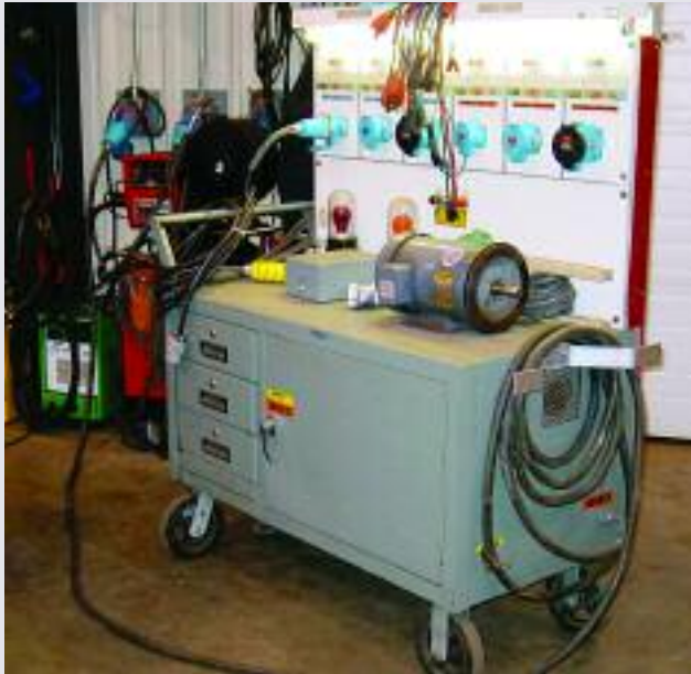
Correct motor rotation can be ensured by pre-testing motors at a test bench with receptacles that match the polarization in the field.
