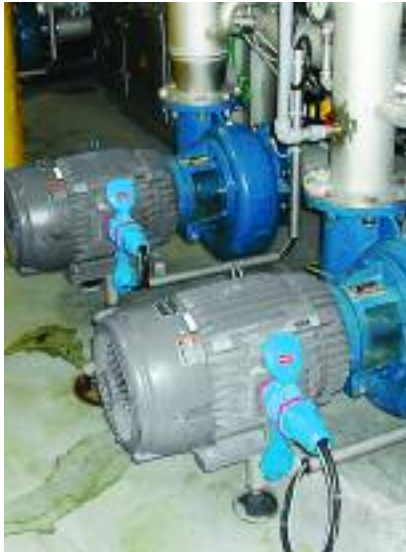
Process Pump Connections
