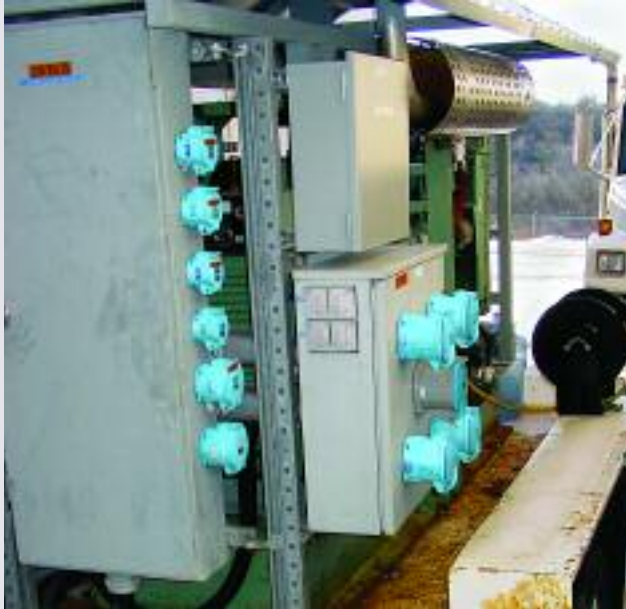
A mobile diesel generator supplies power via Meltric plugs & receptacles during outage conditions.
