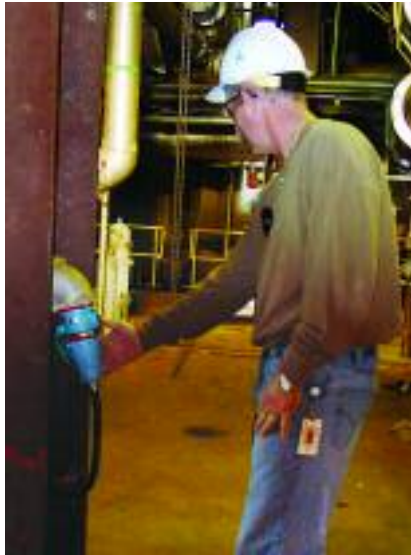
Portable Equipment Connection
