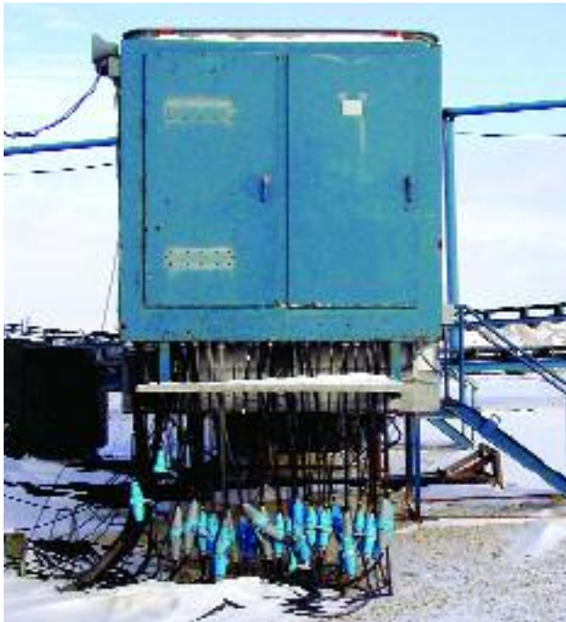
In-line connections are preferred at this quarry to solve a mounting space problem.
