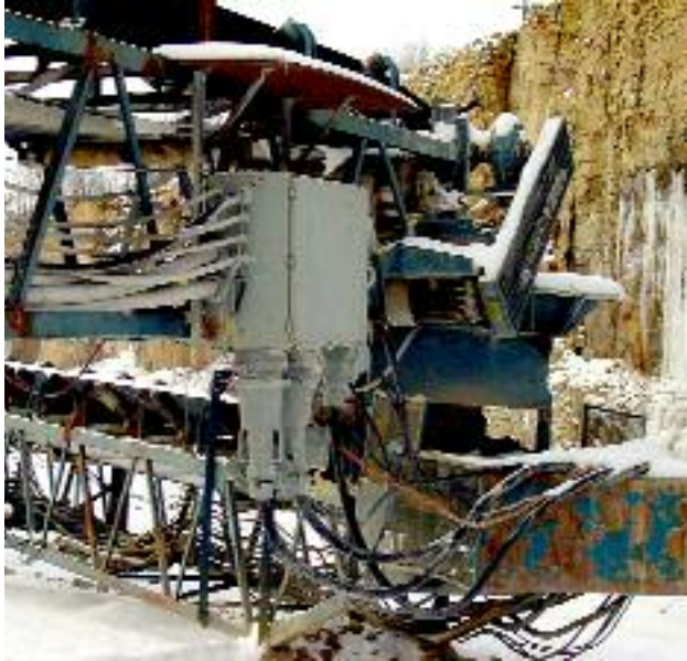
Power to a 500 horsepower crusher motor is supplied by parallel phasing of two 400A PF plugs and receptacles.
