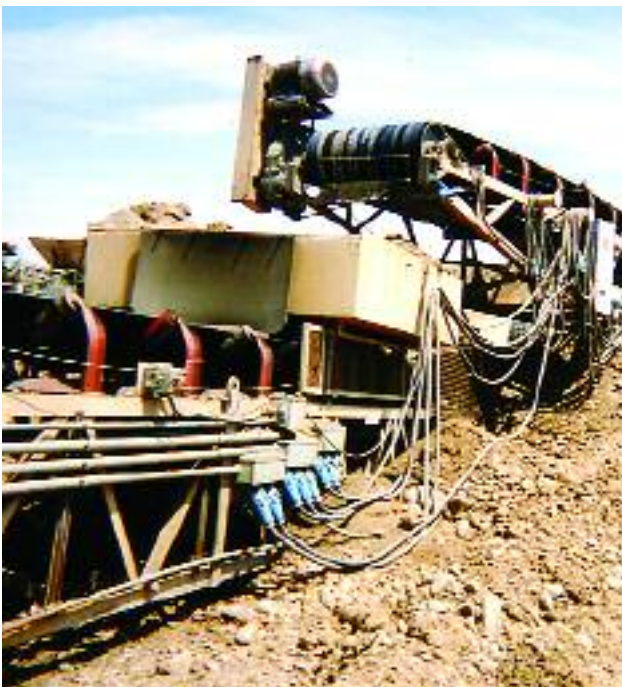
100A DS100's connect motors along a conveyor line.
