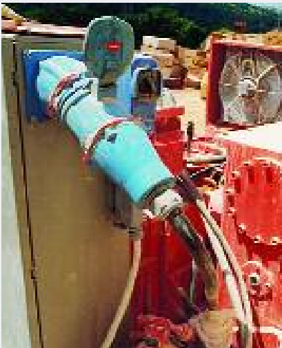
Power connections to a marble cutter
