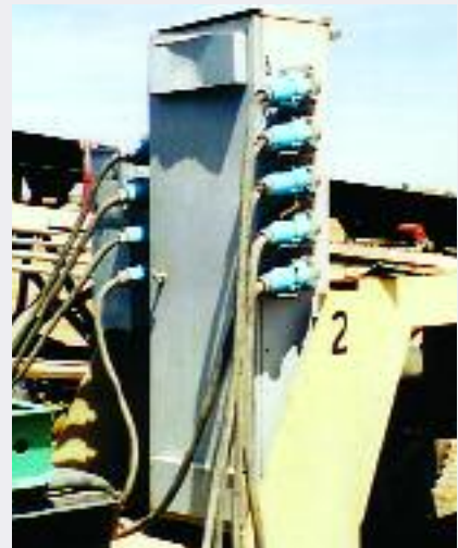
Mobile power distribution panel
